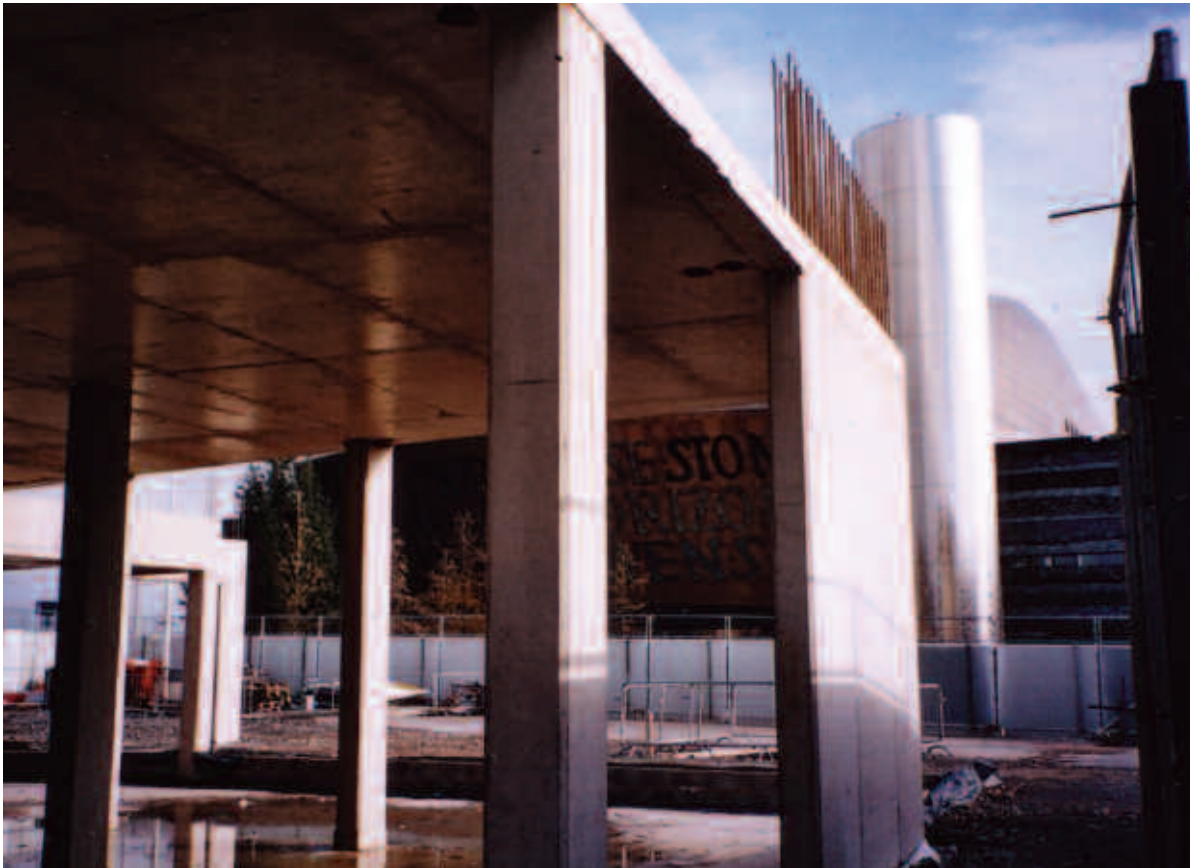
Symbol of the recession: Bellway's 17-storey office block in a prime position facing the Millennium Centre in Cardiff Bay has been mothballed, with building work halted at the first floor.
